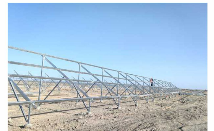
Turpan, Xinjiang PV Project Management Department-PV Support Structure Procurement Project
